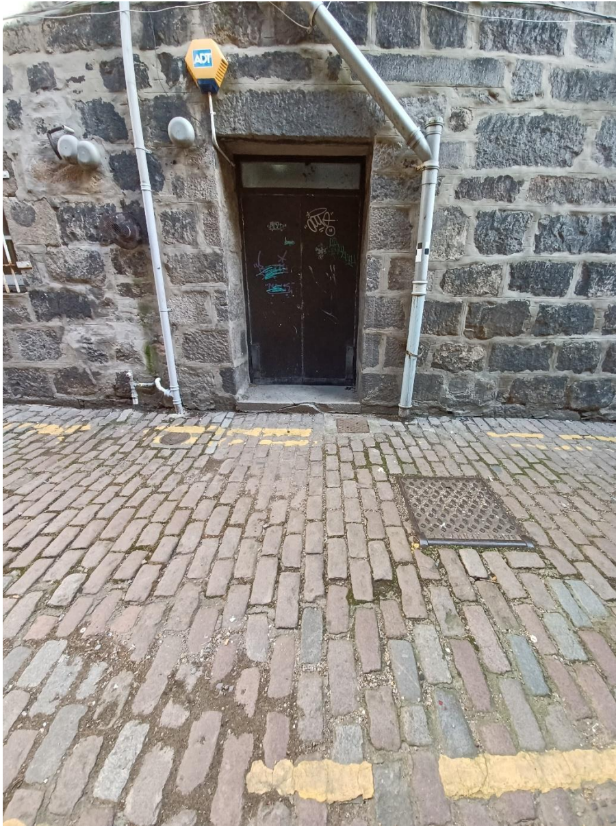
2. Rear door to be replaced
